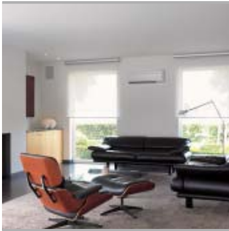
< Wall mounted unit
