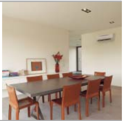
Wall mounted unit >
